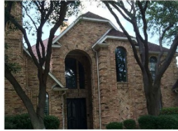
The roof massing is too complex. Openings are not proportionate.
