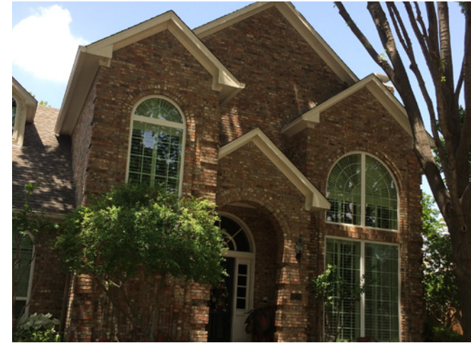
The openings are too large for the home. The massing is too complex for the width of the front façade.
