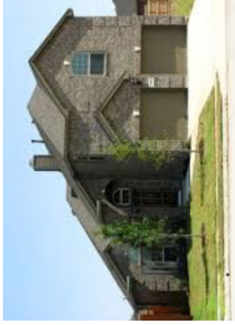
The garage is most prominent and creates disproportioned overall massing. Vent stacks are visible from the street.
