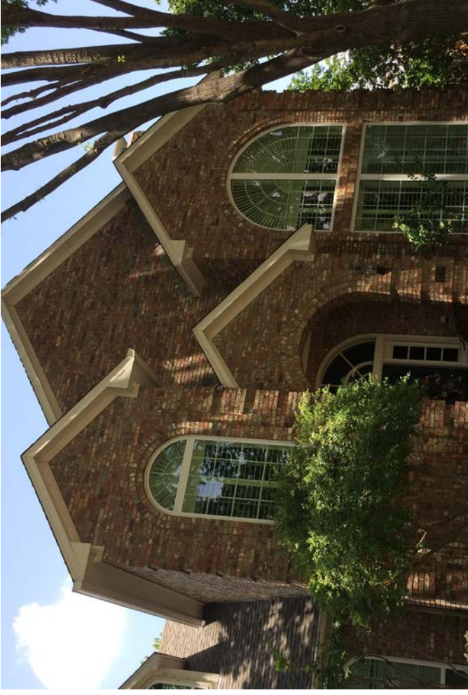
The window openings are too large and out of proportion for the façade. This home has a complex massing where the gable elements are competing for importance.
